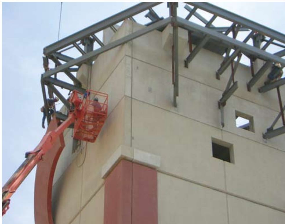
Assembling the top of the tower required detailed planning, complicated rigging and skilled crane work due to the use of sloping panels, canted arch pieces and structural steel angle attachments 100 feet in the air. Photo: Sidley Precast Group.
