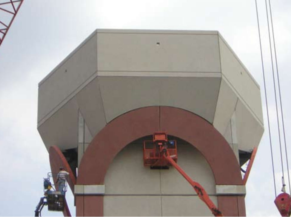
The hexagonal structure appears to rest on canted, precast arches atop a red-accented beige shaft. Photo: Sidley Precast Group.
